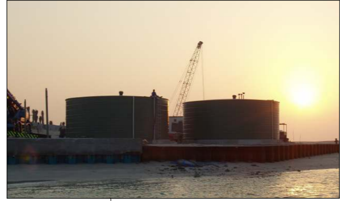
▶ 1 million Ltrs. Installed at World Island project, Dubai.
