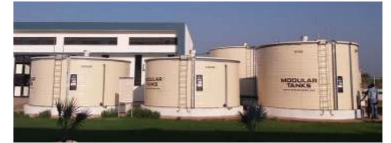
Over 1.2 million Lts. Installed at a Project in Mehsana, India.
