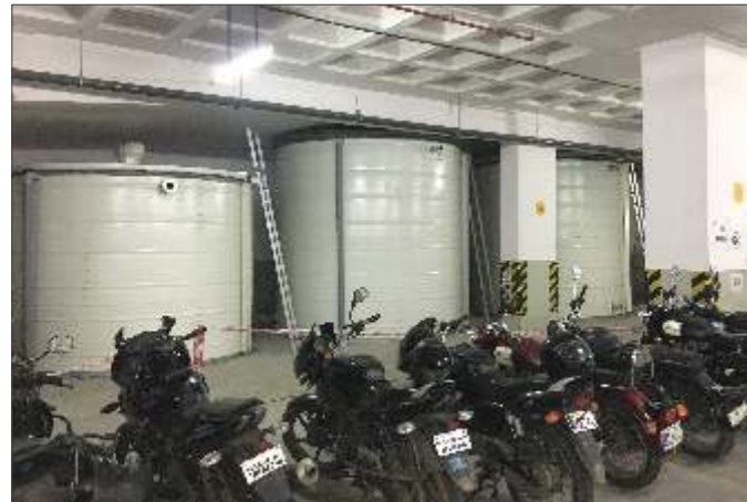
25 KL & 50 KL- 10 Nos. Installed at a Project in Bangalore, India
