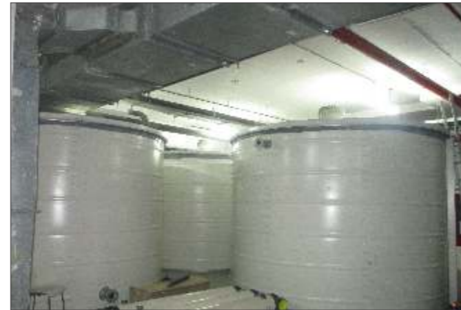
38 KL & 55 KL- 7 Nos. Installed at a Project in Bangalore, India
