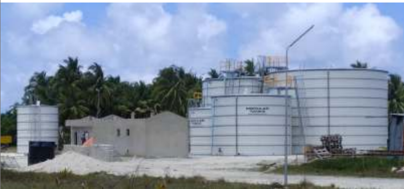
300 KL-3 Nos + 100 KL Installed at a Project in Bangalore, India
