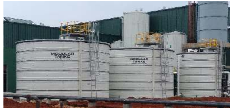
4 million Ltrs. Installed at a Project in Maldives
